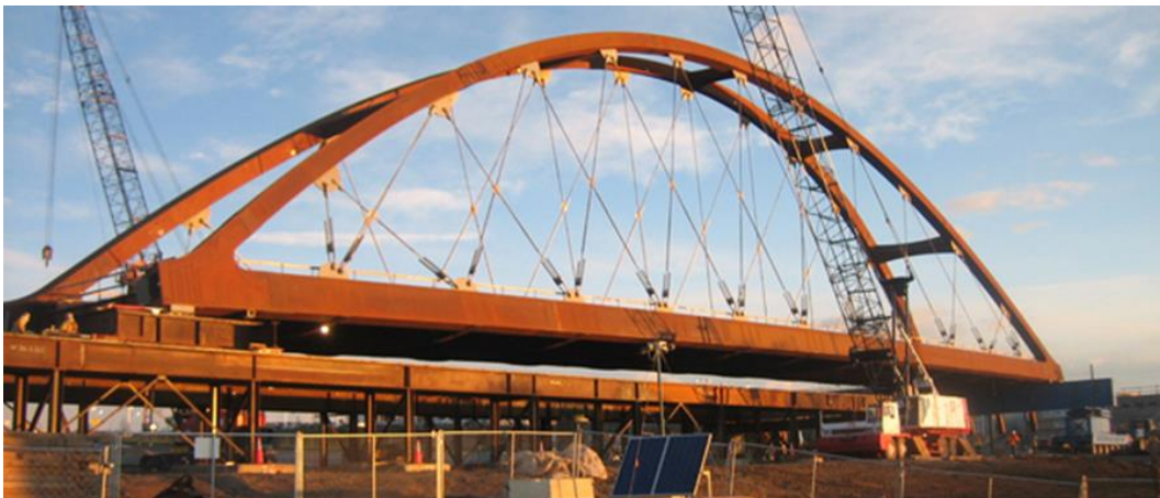
Figure 17 Tied Arch Bridge Slide. Hydraulic jacks to left, SPMTs to right of image.
